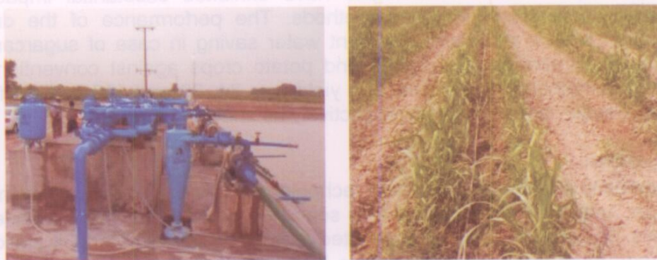
Figure-5: A view of installed drip irrigation system for sugarcane (district R. Y. Khan)
